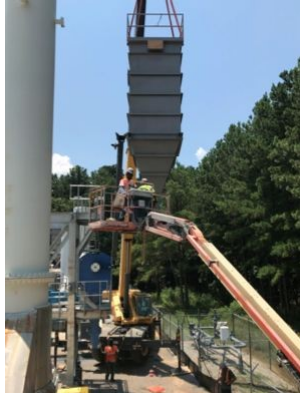
Work crews install one of four new bag houses (grey item) at the Lauscha Fiber International plant in Summerville. Officials with plant's parent company, Unifrax, said they expect the equipment fixes to prevent additional unexpected fiber releases in the future. Contributed/Unifrax
